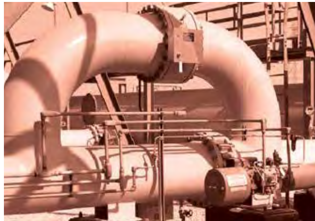
API 537 Compliant Application
